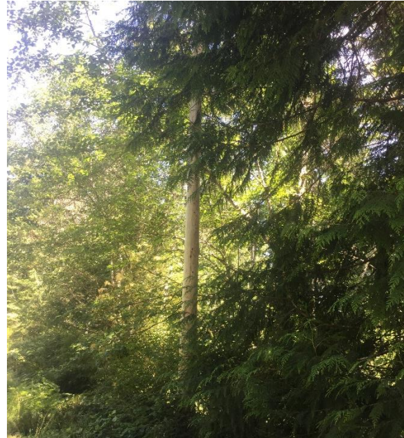
Figure 1. Vegetation encroachment on powerline- Cortes Island.
