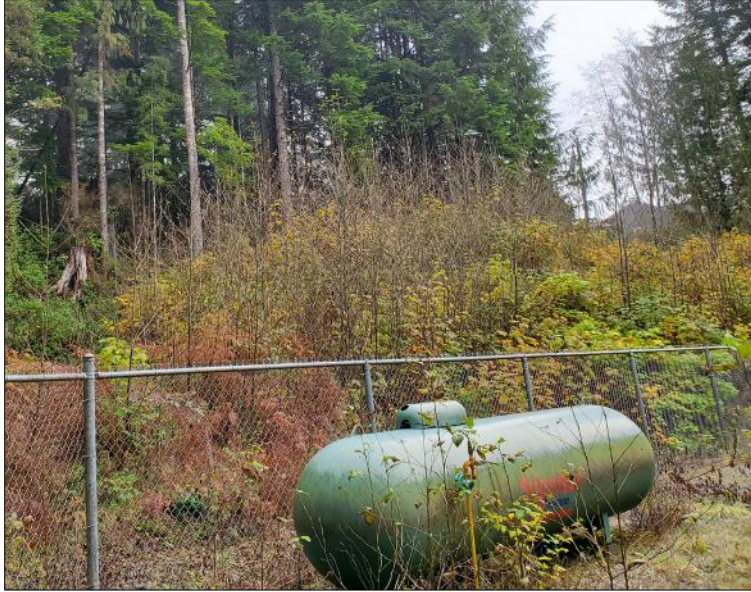
Photo 4. Propane tank serving as the back-up power source for the water treatment facility.
