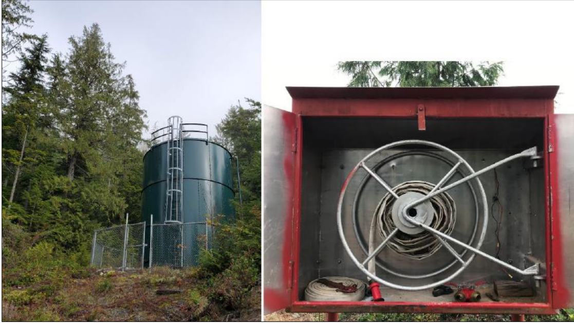
Photo 3. On the left: the water reservoir (tower). On the right: one of four fire hydrant hose boxes.
