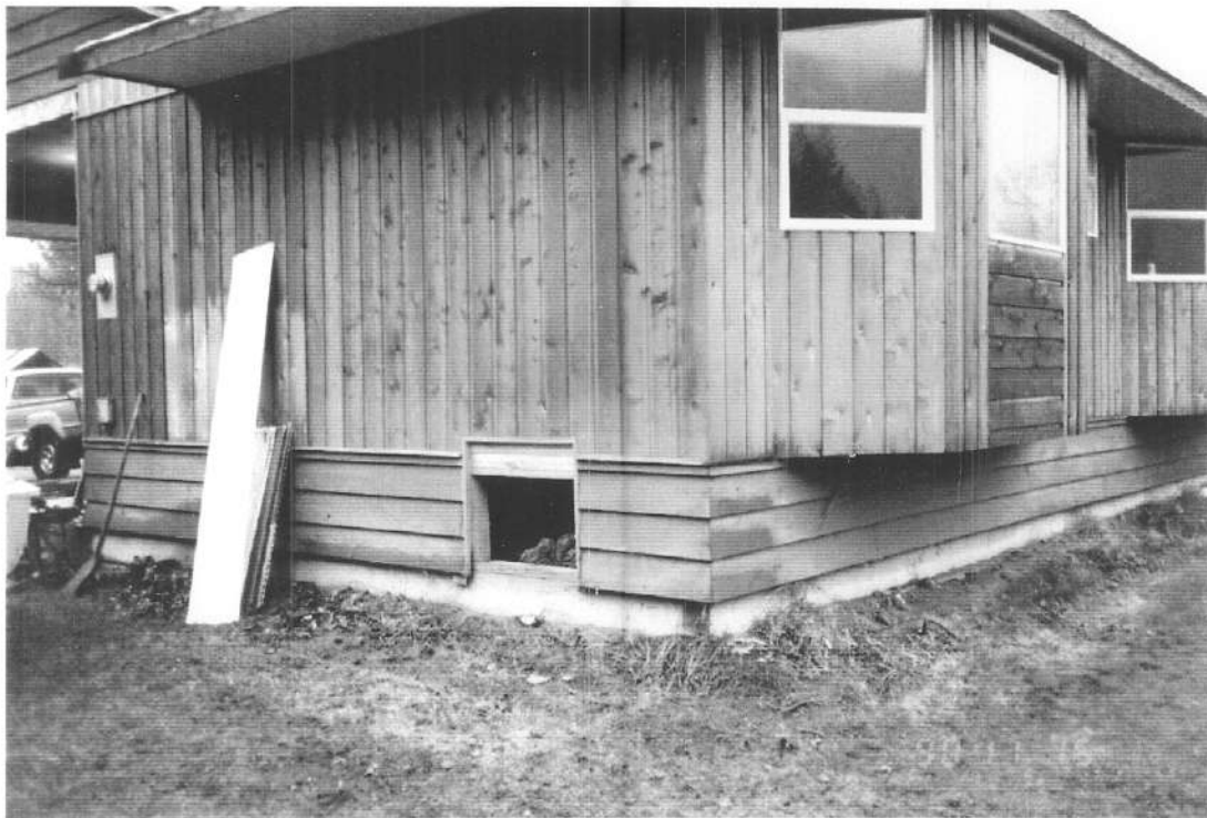
PHOTO 3: HWM 90-29 - TOP OF FRAME AROUND ACCESS DOOR - HOME LOCATED AT THE FOOT OF ARMISHAW ROAD (NOTE THIS HOME WAS FLOODED DURING THE 1975 EVENT AND SUBSEQUENTLY RAISED ABOUT 2 FEET)
