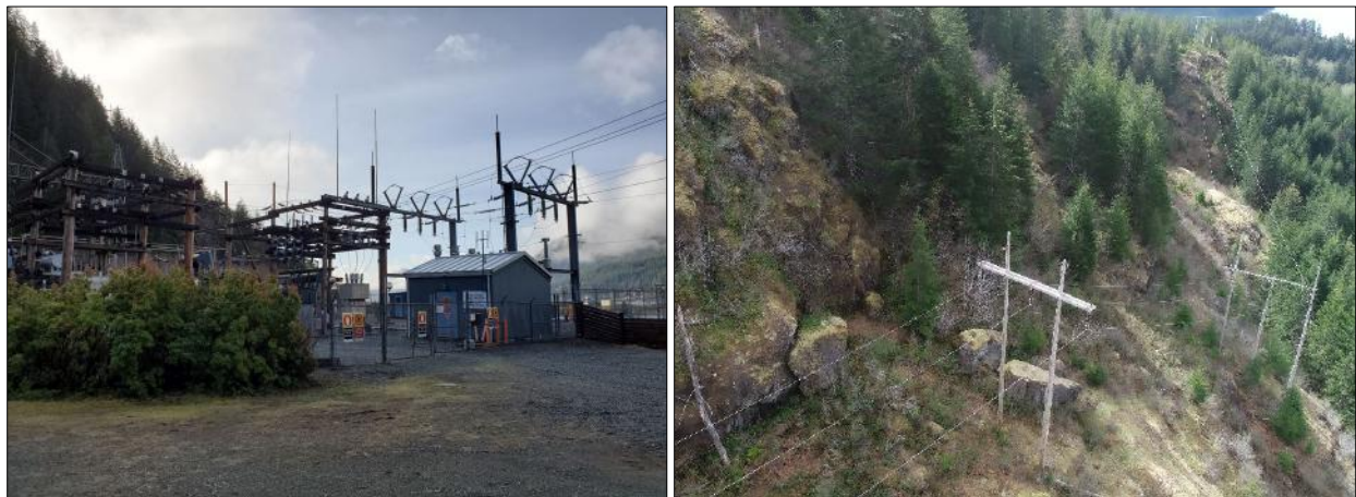
Photo 3. The BC Hydro substation is located adjacent to the single access road in/out, Head Bay FSR. Wooden poles are the supporting system of the cables.
