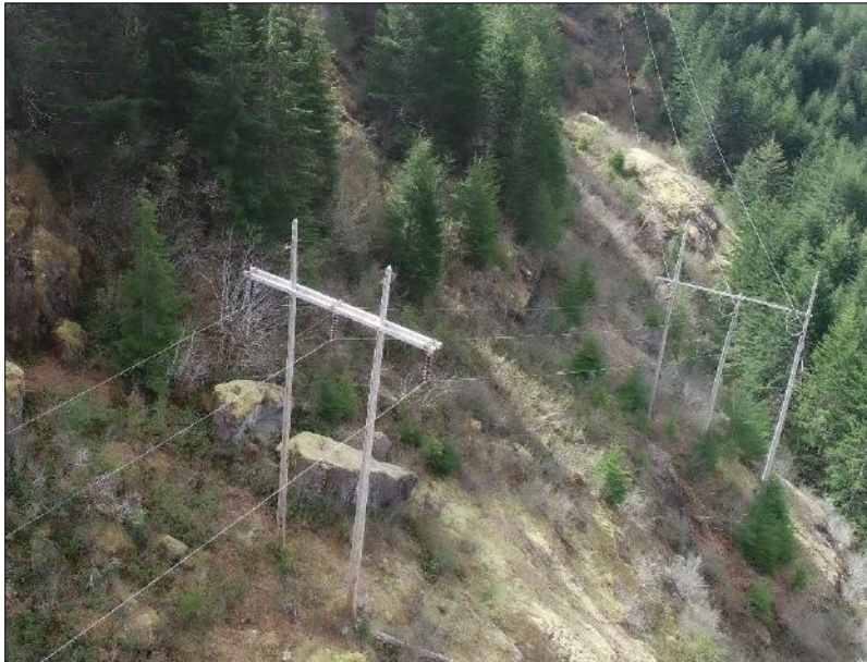
Photo 3. Wooden power poles running into Zeballos.
