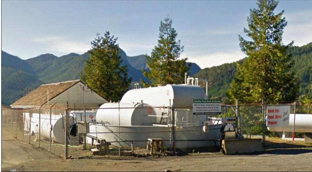
Photo 7. Fuel storage tanks at the Zeballos fuel dock.
